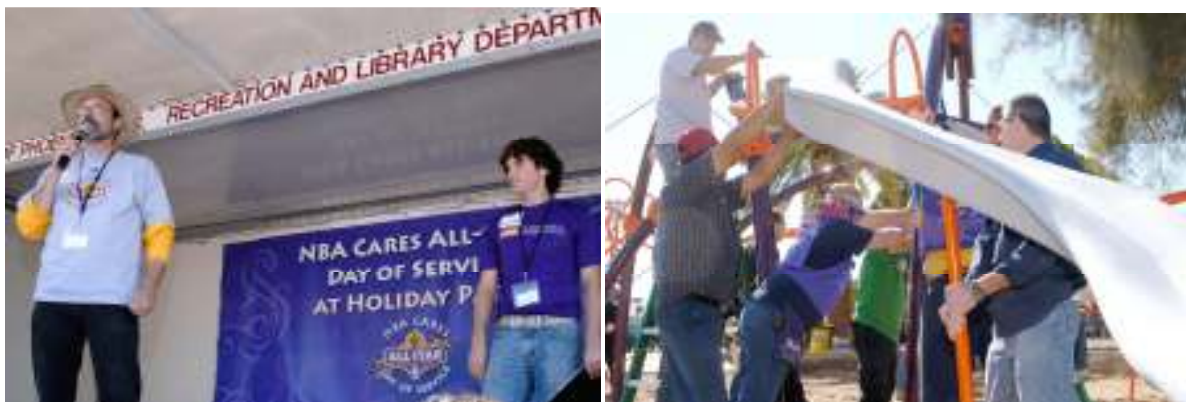
Working with NBA All Star Game Volunteers Installing Playground at Holiday Park.
